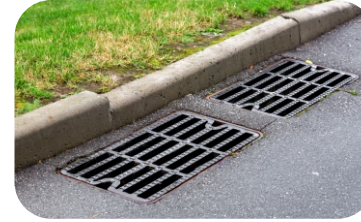
Storm Water Drainage
