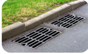
Storm Water Line
