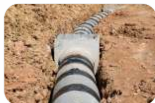
SEWAGE PIPE LINE
